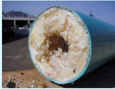
Pipe clogged with FOG
