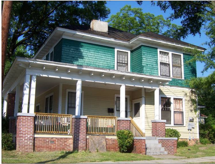
This house exhibits a variety of wood sheathing, trim, and ornamentation. Clapboard, paired porch posts, wood shingle siding, decorative cornice, and window surrounds are all made of wood.
