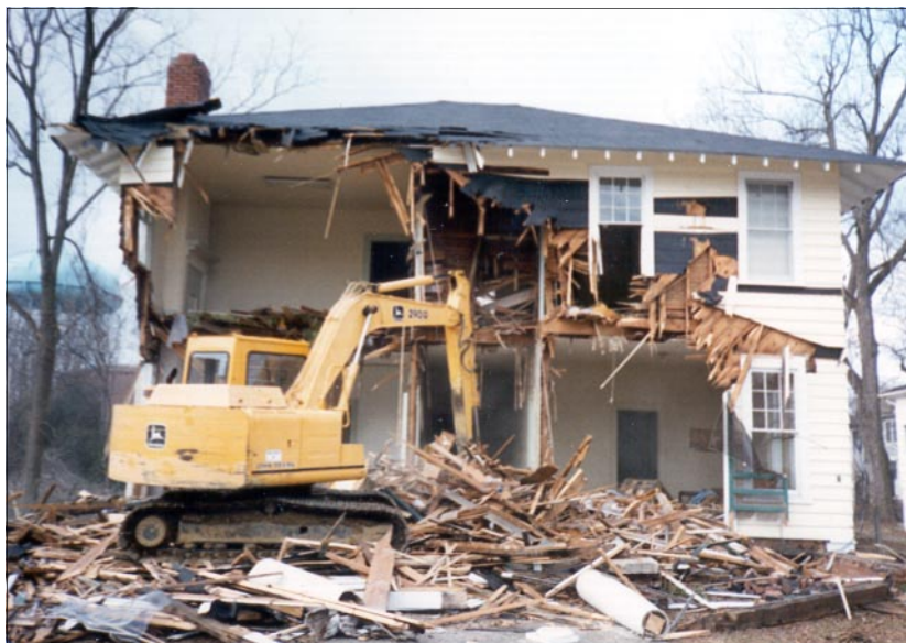
Demolition of Wilson's historic buildings is inappropriate to the character of historic districts and local landmark properties.
