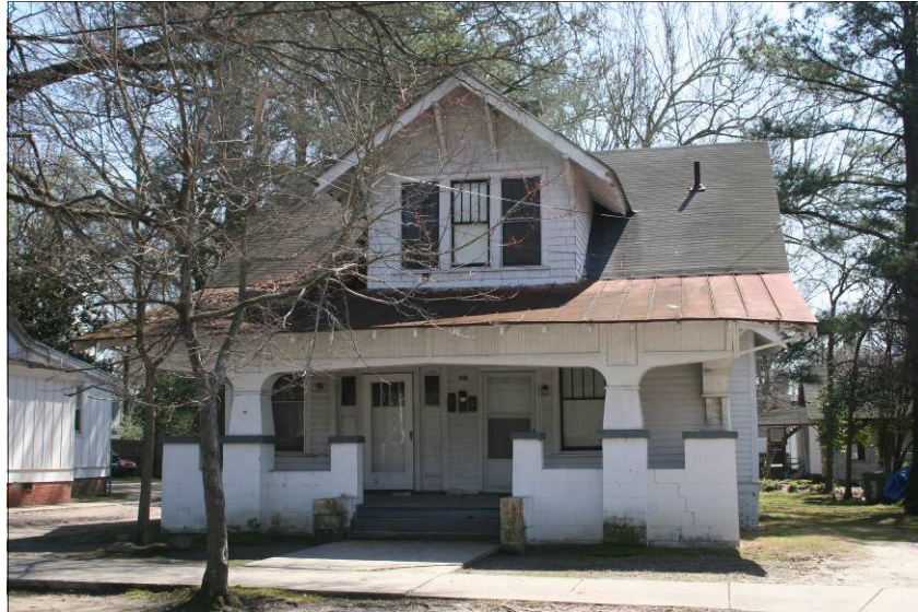
This one-and-one-half story example has a broad, side-gable roof, full-width porch with tapered piers and brick plinths supporting a paneled shallow arch. The elbow brackets, exposed rafter tails, Craftsman-style windows, and wood shingles are also character-defining features of this bungalow.
