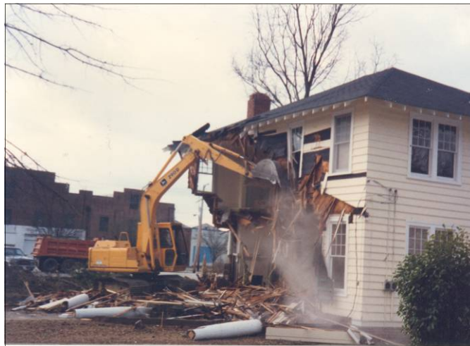
Demolition of historic buildings causes unsightly voids in the historic streetscape and districts and removes an irreplaceable part of Wilson's history.
