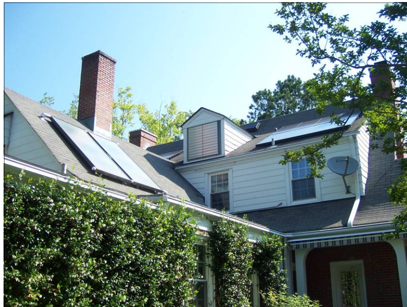
The solar panels on this home are flat and on the rear elevation within the tertiary AVC so that they are not visible from the public right-of-way.
