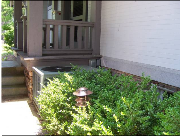
This HVAC unit is well-screened from public view.
