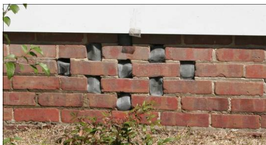
Example of pierced brick vent in brick foundation with screen installed for rodent protection
